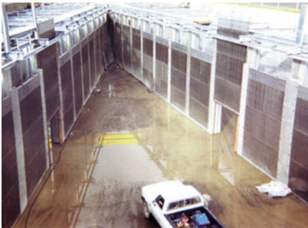
Chevron Intake in the Dry
