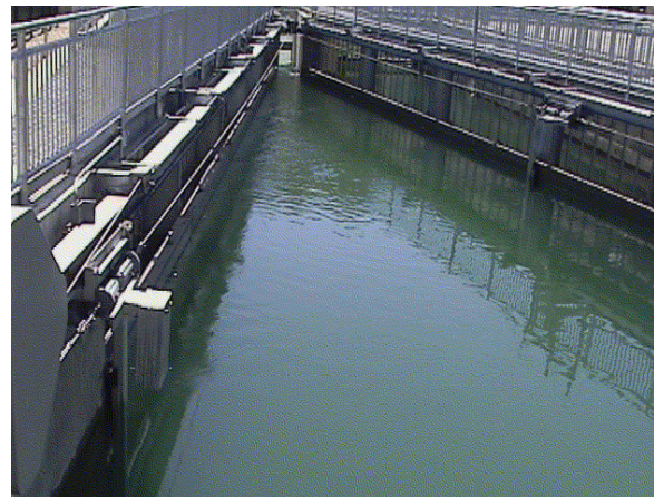
Chevron Intake in Service
