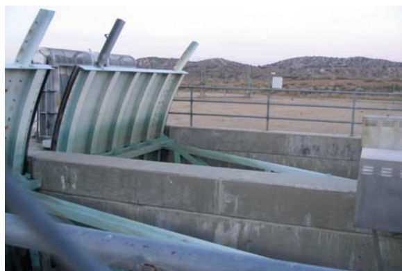
Radial Control Gates on the California Aqueduct
